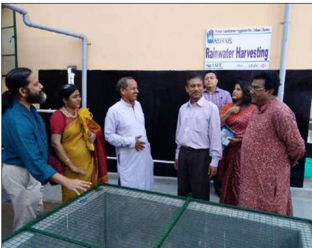
Rainwater harvesting system at WASH-US site
