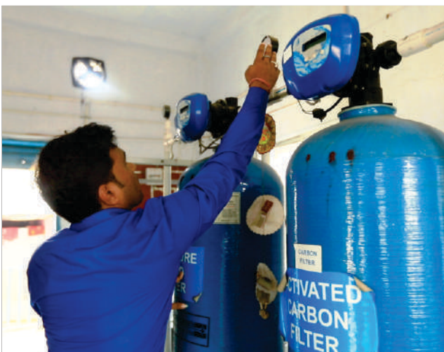
Water purification system
